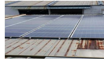
Sri Kembangan, 8.7 kWp
